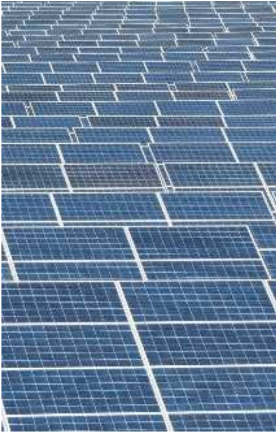
Solar photovoltaic panels
